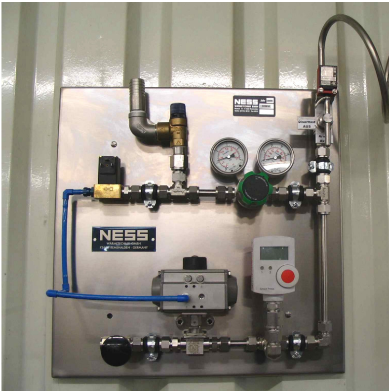
Picture 1: Ness fire extinguishing systems for thermal oil heaters.
