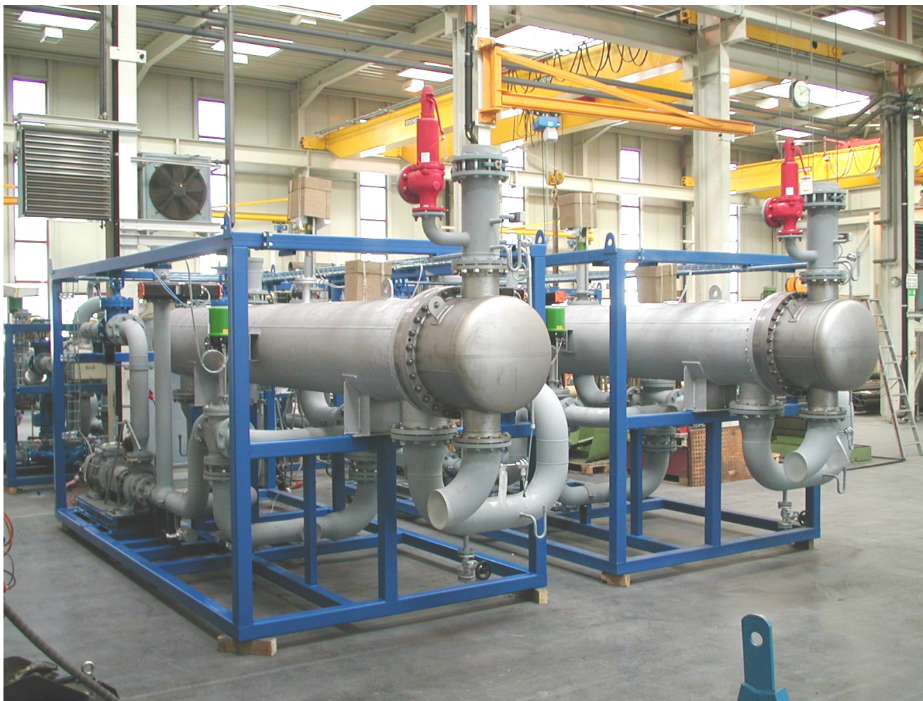
Picture 2: Hot water - heating- and cooling system
