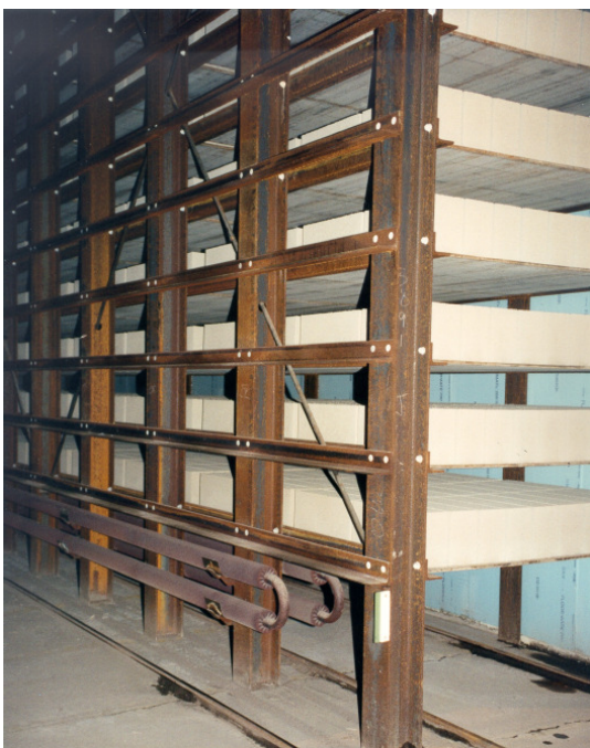
Picture 1: Thermal oil heating register in a concrete block chamber
